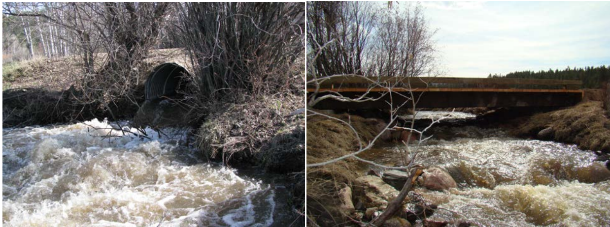
Photos 1-2: Undersized culvert replaced with a free-span bridge on Willow Creek near Lincoln, Montana.
